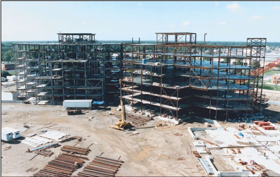
The current Defense Logistics Agency Weapons Support (Columbus) headquarters building is under construction Aug. 10, 1997. DLA's first foray into Office of Management and Budget Circular A-76 public-private competitions after a post-Cold War hiatus examined its bus and taxi service at Defense Supply Center Columbus in Ohio.
